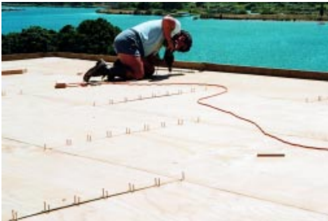
Note: Staggered sheets and screw fixing with face grain running at right angles to the joists.
